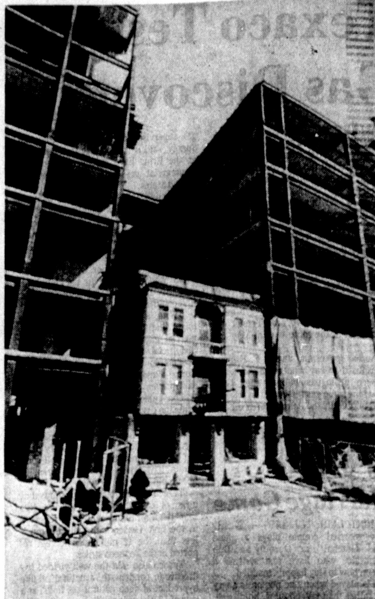
SURROUNDED — Mrs. Vera Coking's 22-room boarding house on Columbia Place in Atlantic City is nearly surrounded by structural steel for Penthouse's casino hotel. Mrs. Coking said construction has hurt her hotel business. (AP Laserphoto)
