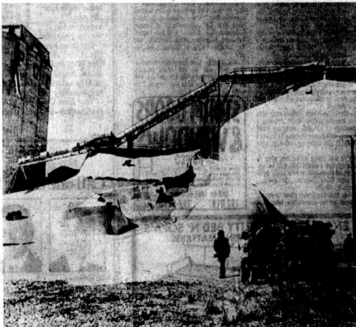
MAMMOTH WHEAT SPILL — More than 18,000 tons of wheat cover the ground around this ruptured grain storage bin in the eastern section of Amarillo after the huge structure split down the middle Monday. The bin, one of three at the Pro-
