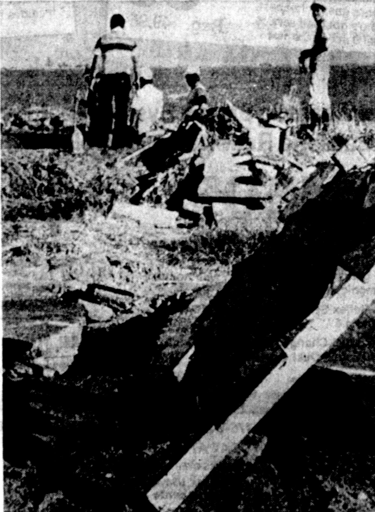
CRACKS APPEAR ABOVE FAULT — Workers repair an irrigation ditch and road cracked above the Imperial Fault which slipped during Monday's earthquake in California. More quakes jolted the area Wednesday. (AP Laserphoto)
