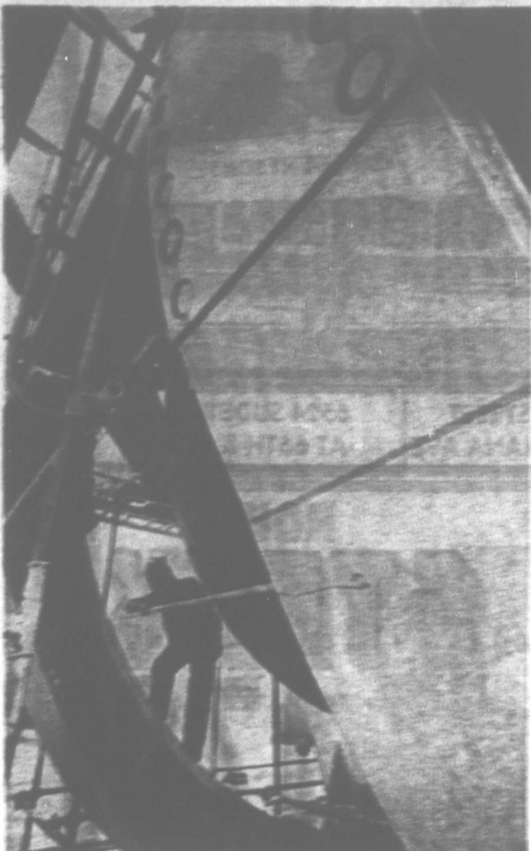
CRITICAL EYE — This steam generator going into the Waterford 3 Nuclear Station of Louisiana Power and Light at East, La., is getting a critical once-over from Marc Alexander Polansky, Mrs. Polansky, the only woman of 300 authorized nuclear inspectors in the country, checks to make sure the generator complies with standards and codes of the Nuclear Regulatory Commission and the American Society of Mechanical Engineers. (AP Wirephoto)
