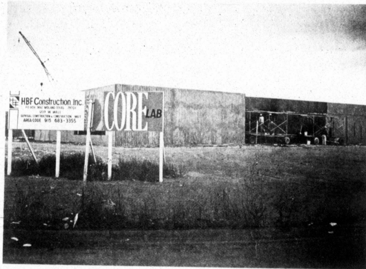
Pre-fabricated walls go up on a 25,000 square foot building to house Core Lab facilities in the near future. The new structure is one of three new industries going up at Midland Industrial Park.
