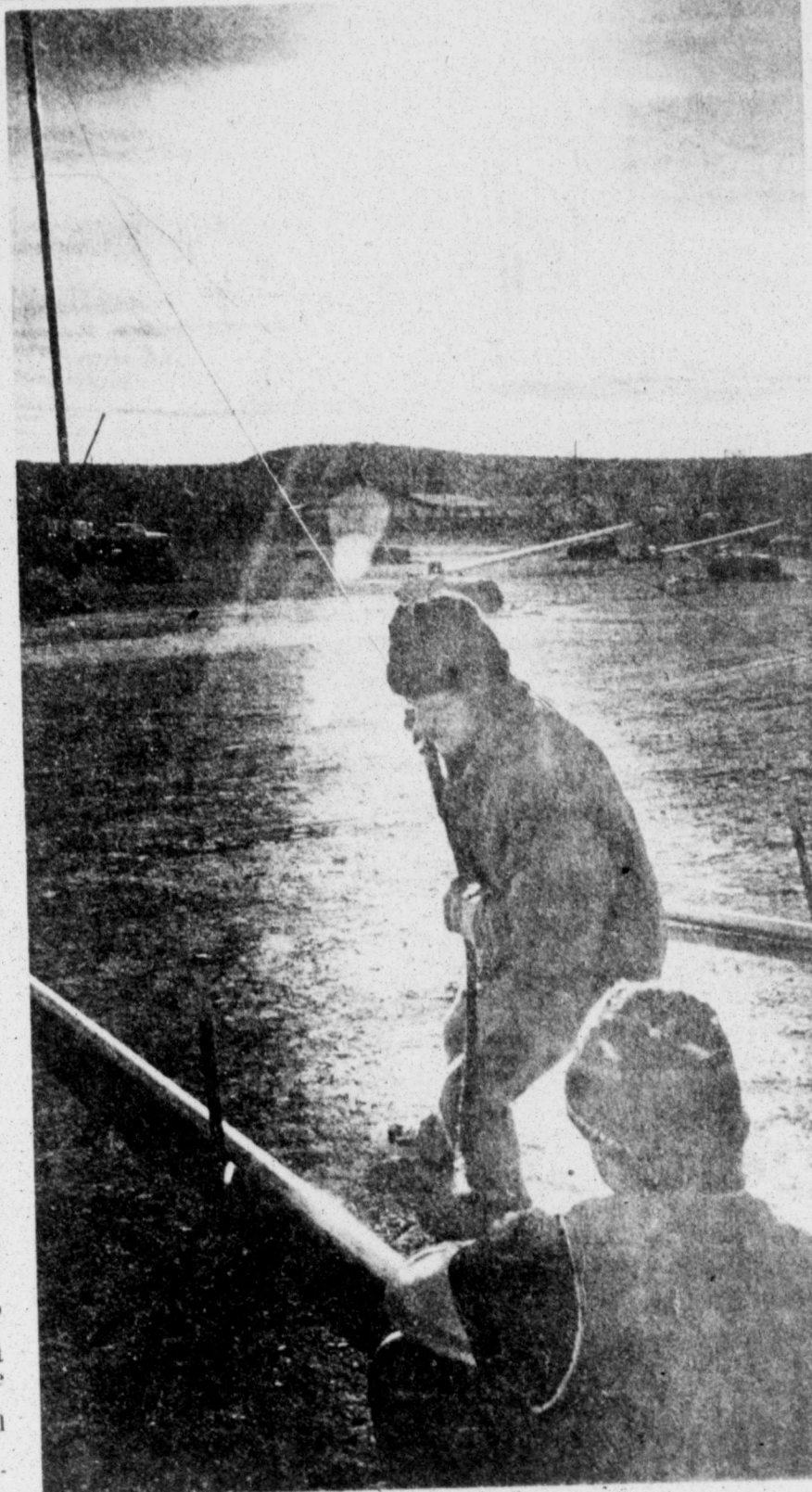
Chilly weather greets technical crews as they begin raising the tent at Big Spring's Howard County Fairgrounds. A worker pulls back on a cable to help center one of four 56-foot main masts, while the other waits to tie the line.
