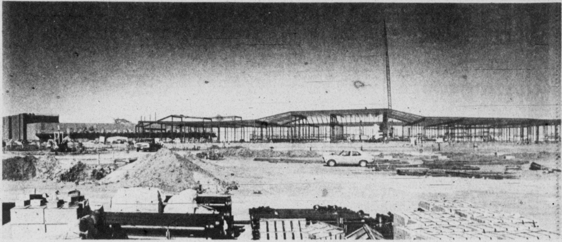
Steel beams stretch toward the sky as the 750,000 square foot Midland Park Mall continues right on schedule, say developers Melvin Simon & Associates of Indianapolis, Ind. Walls planned for the late spring of 1980. (Staff Photo by Mike Kardos)
