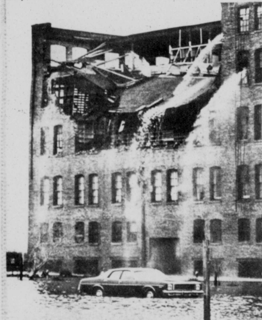
Winds from Hurricane Frederic ripped a hole in the side of this large building in Mobile, Ala., Thursday morning. Streets were flooded and most residents were without power due to the fury of the storm. (AP Laserphoto)
