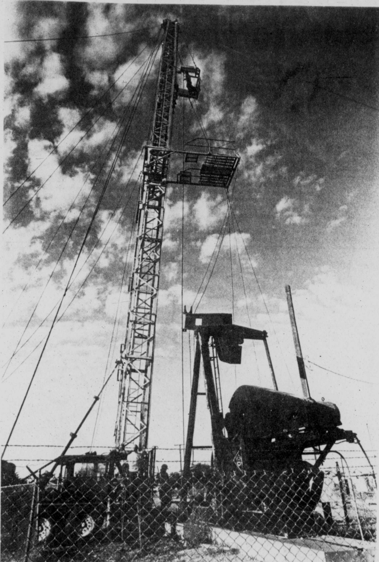
Workers replace pumpjack rods at the No. 1 Inez Fasken oil well owned and operated by Miller Exploration Company of Midland. Located in the 100 block of South Eisenhower Drive, the well reportedly is the only producing one within the Midland
