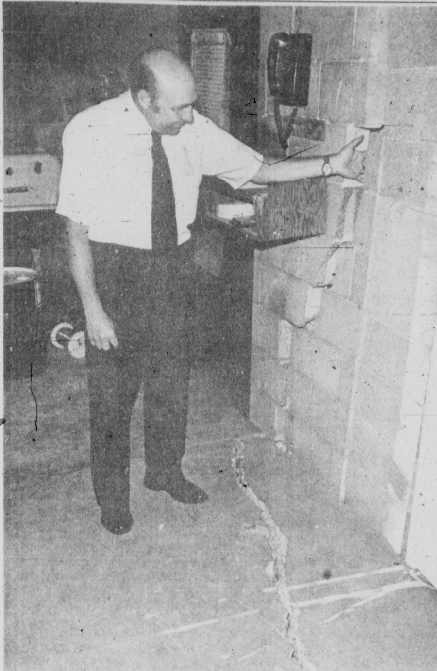
Director of Public Works Fred Baker inspects cracks in the walls and floor of the Service Operations Building. The cracks have been caused by the building — which was constructed over an old landfill — having sunk about a foot. (Staff Photo by Bruce Partain)
