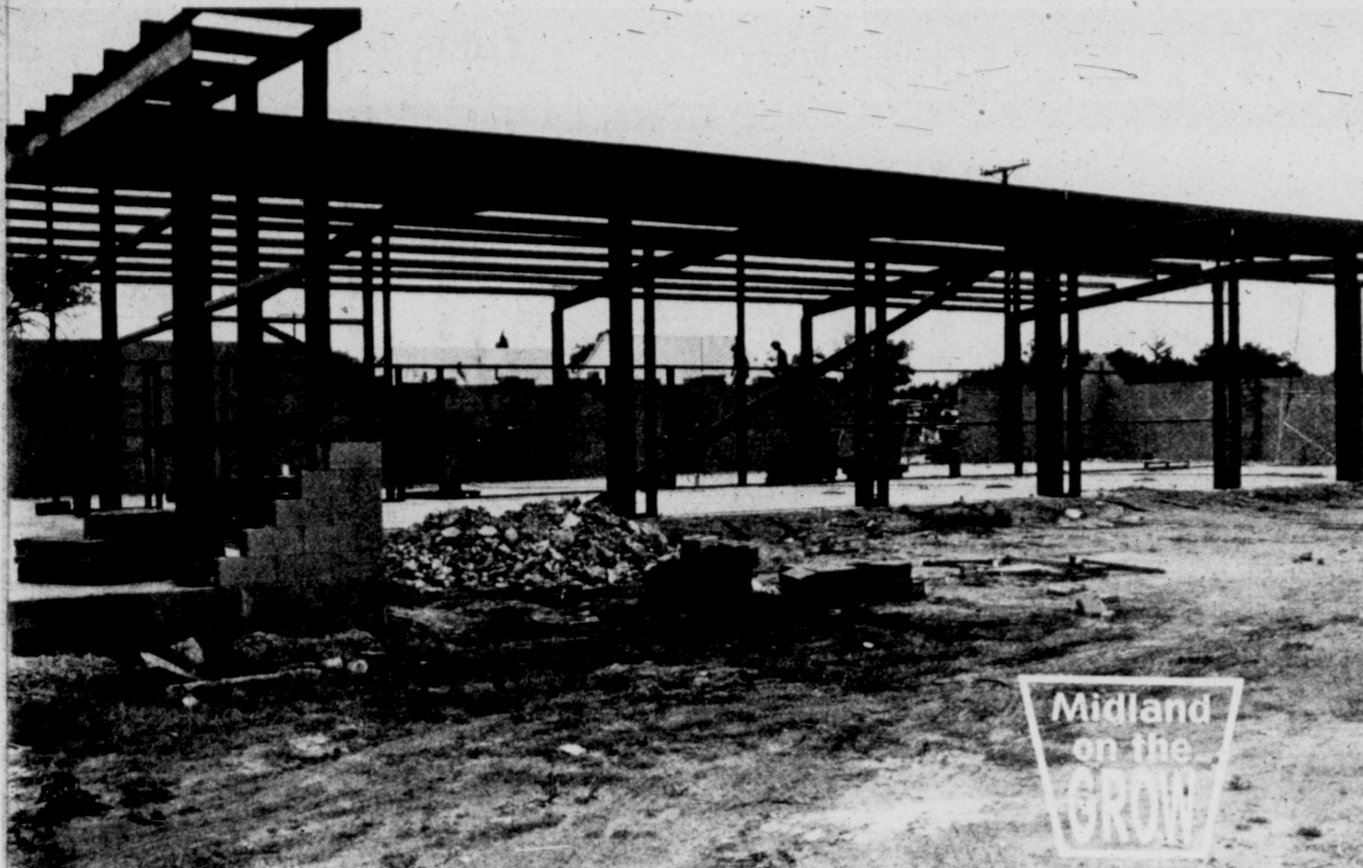
Cinder block walls of the new Balie Griffith-Firestone Inc. store in the 700 block of North Big Spring Street are being mortared in stair-step fashion next to the steel girders. The building is expected to be completed before
