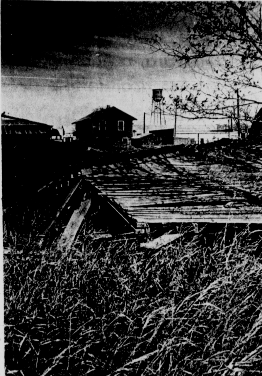
The past fades and edifices of yesteryears — such as this "exhausted" building in Stanton — collapse. Stanton once carried the place names of Grelton and Marienfeld. (Staff Photos by Ed Todd)
