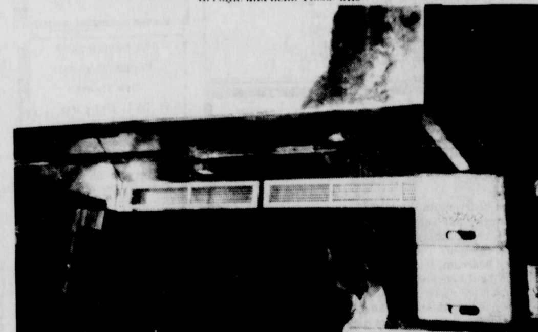
NEW KITCHEN AREA: A worker for Earl Thompson Construction Co. is shown in the above photo putting in the Vent-A-Hood for the kitchen area. The new cafeteria will also have a stage for special performances. (Staff Photo)
