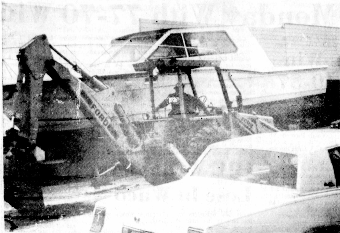
WATER LEAK — Although there was water leaking through the pavement along the 700 block of Conrad Hilton Avenue last week, a boat was really not needed in order to go down the street. City crews brought a backhoe to the area and started efforts to repair the leak in the
