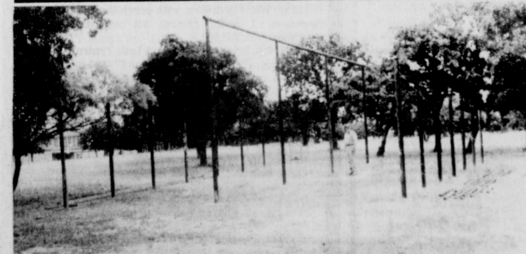
STEEL FRAMEWORK for a large picnic pavillion is near completion at City Park as the above photo shows. Members of the Cisco Lions Club (noon) are erecting the pavillion and Chairman Bob Conner is shown in the picture. Much of the material for the project has been donated and, to date, all labor has been donated by club members. - Staff Photo.
