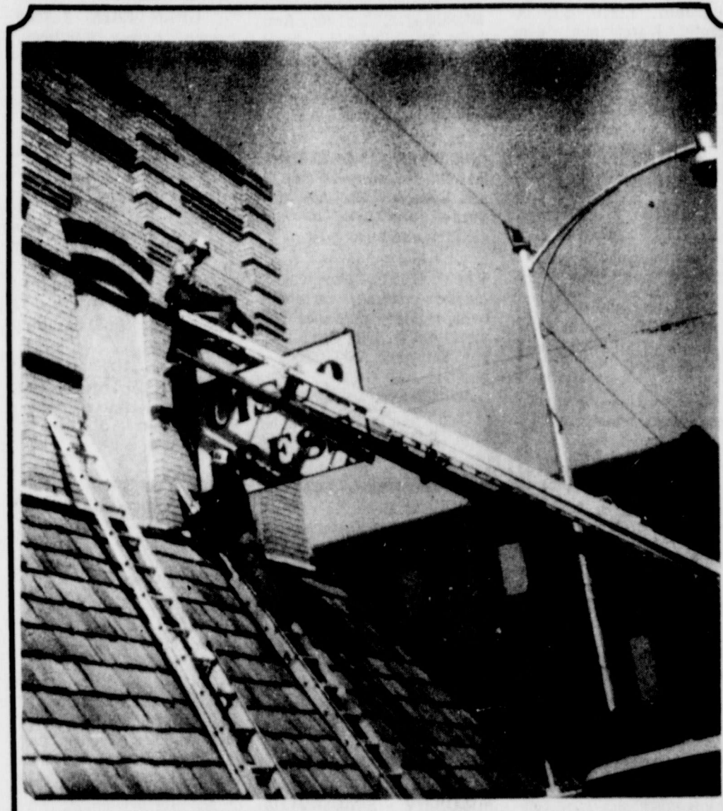
NEW SIGN GOING UP - A new sign was going up at The Press building in Cisco when the above picture was made Tuesday. Herrera Sign Co. of Eastland made the sign and installed it. Richard Herrera of the firm is shown on the lower ladder and his son, Ricky, is atop the sign attaching it to the building. - Staff photo.
