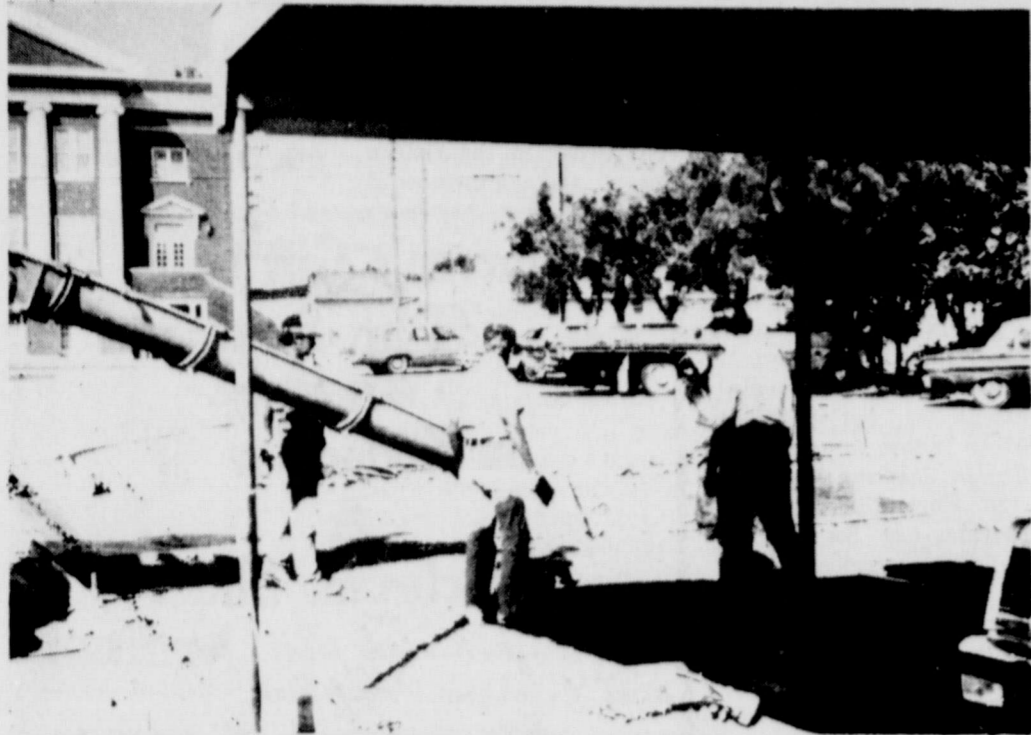
Construction is underway for two new hand-operated car wash stalls at the Robo Carwash, on the corner of Avenue D and 9th. Above, left to right, Randy and Ollie Moran, pour cement for foundation as Don Wallace, contractor for the job, looks on. The job should be completed in two to three weeks. Watch for announcement in the Cisco Press. (Photo by Helen Wallace)
