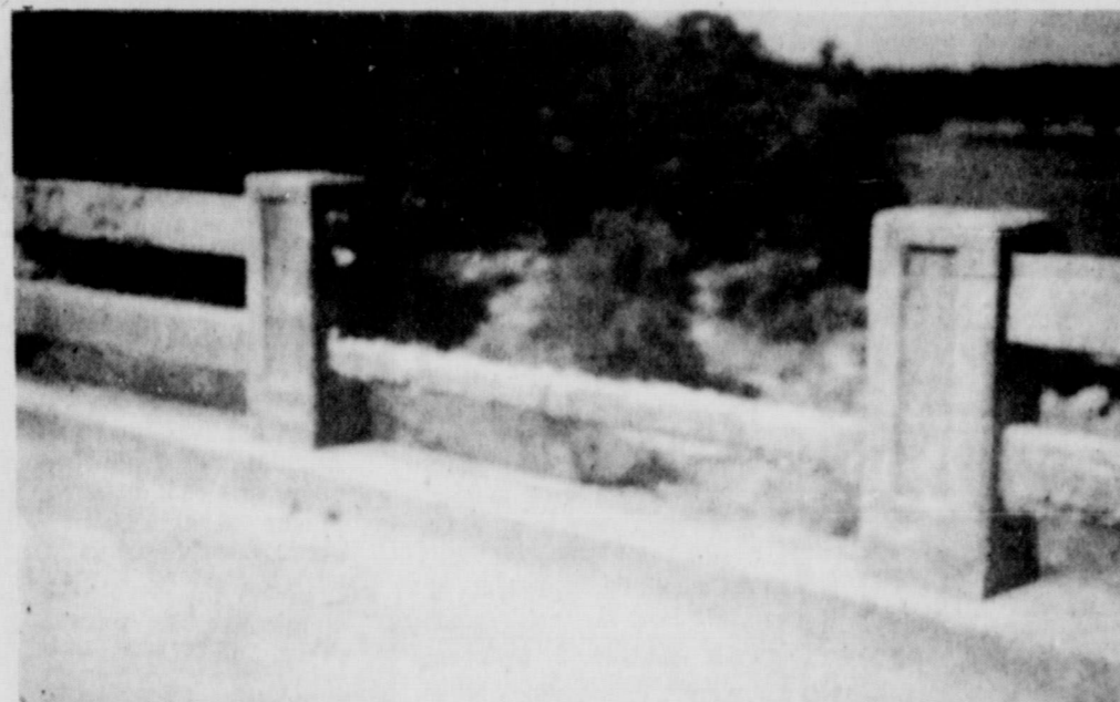
THE LATEST vandalism at the Lake Cisco Park area, according to City Manager John Boland, is shown in the above photo. Mr. Boland said the crossbar on Williamson Dam has been knocked out by a sledge hammer and persons have been using the opening for a place to dive into the lake. He went on to say such vandalism is the reason Lake Cisco Park is to be closed from sundown to sunup and also why the city is attempting to close off the bridge which crosses Williamson Dam.
