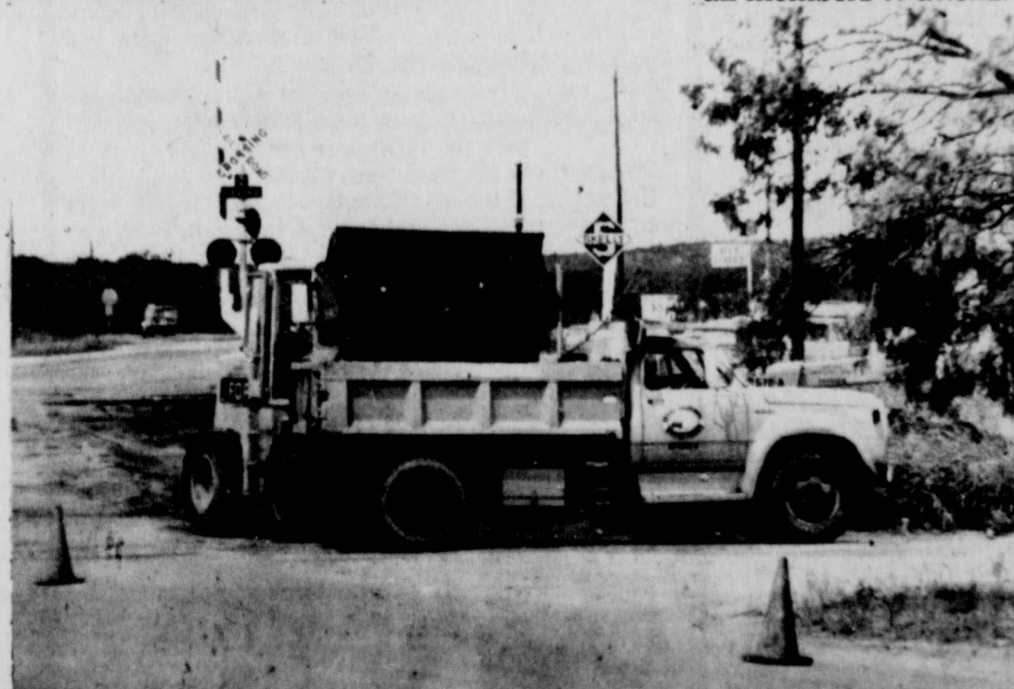
TEXAS HIGHWAY Department crews were working on a bad drainage area in Cisco Friday next to the railroad tracks which cross the north end of Avenue D. During heavy rains the area almost becomes a small creek. Plans also call for the state crews to re-blacktop Avenue D from the railroad, south to 8th Street. (Staff photo)
