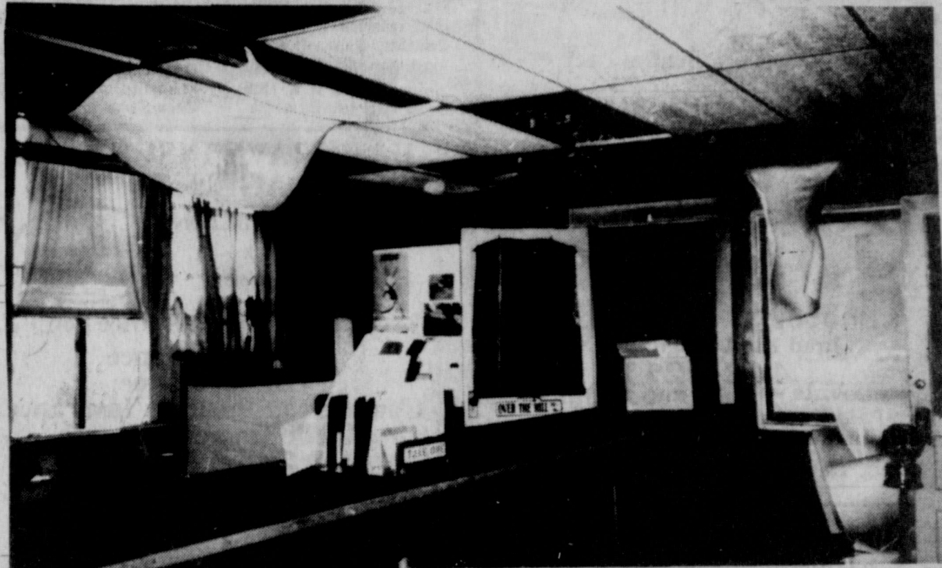
DAMAGE TO the offices at City Hall was extensive as the above picture shows. City employees moved into temporary quarters at
