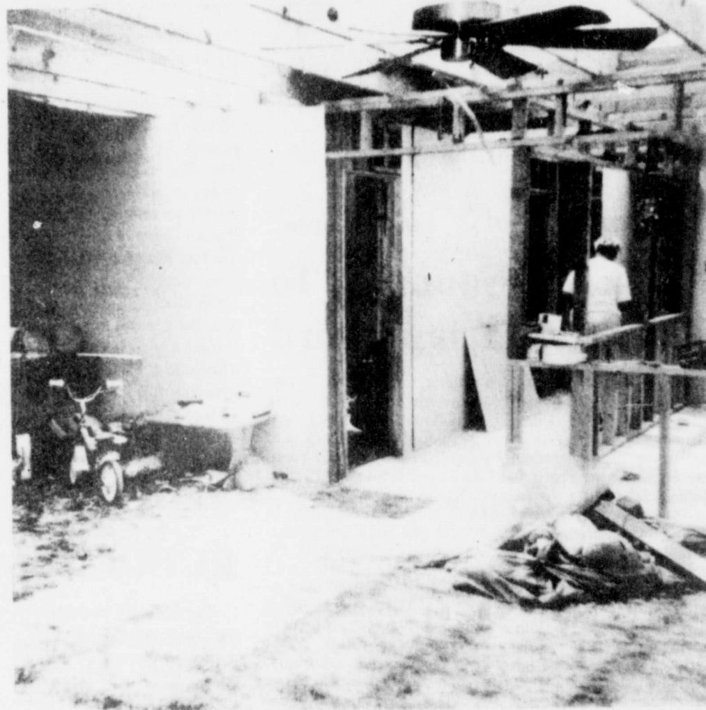
The inside of the McCurry home without the roof and with some of the sheetrock missing.
