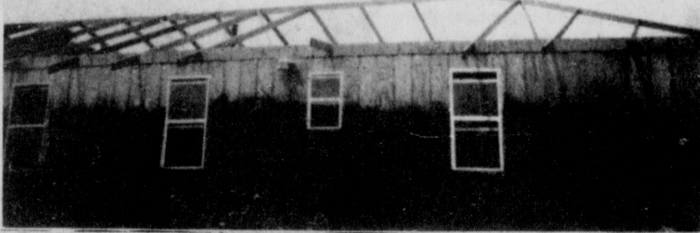
The outside view of the McCurry home after a tornado ripped the roof off Tuesday night.
