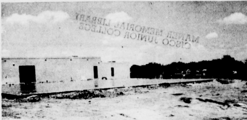
CEMENT SLAB-- The cement slab for the new Physical Education Gym at the Cisco Elementary School was poured last week, ready for the building to begin. The P.E. facility will be ready for use by the students in September. (Staff Photo, courtesy of Cotton's Studios)
