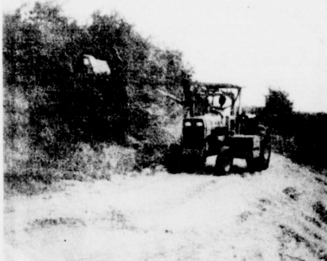
Fred Hull operates an automatic tree-trimmer on a rural road south of Cisco. This is part of the road equipment in Pct. 4. The automatic trimmer saves a lot of labor, according to Billy Bacon, Commissioner of Pct. 4.
