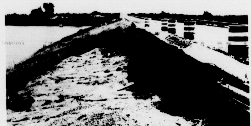
Dam slippage-erosion is still very visible at Lake Leon dam.
