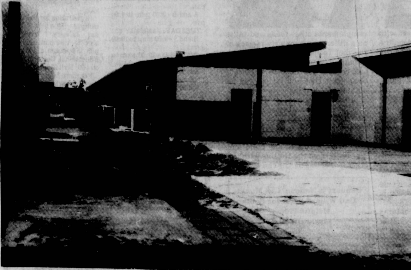
WORK HAS BEGUN at the Cisco Elementary School over the holidays on Phase II of the new School Building. The part shown in the above photo is where the principal's office was. Mr. Lindsey and Mrs. Puryear will use offices in the
