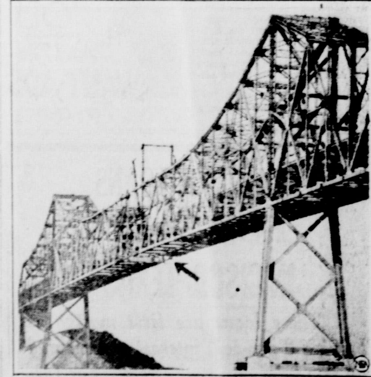
Clinging to girders and dangling from cables, workmen in the upper photo appeared like flies as they completed the difficult job of "hooking up" the last arms of the world's largest cantilever bridge, the San Francisco-Oakland Bay span. Working on their precarious perches, the bridge crews hoisted two huge eyebars simultaneously and fastened them with pins weighing several tons each. In the lower photo the bridge is shown after the last gap had been closed, the arrow pointing to the juncture. Traffic will flow east from San Francisco across the tandem-suspension bridges, through the Yerba Buena tunnel, and across this cantilever span, 185 feet above high water.
