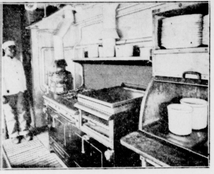
T. & P. new air cooled diner kitchen showing water heaters, range, griddle, and portion of steam table fired by stargas.
