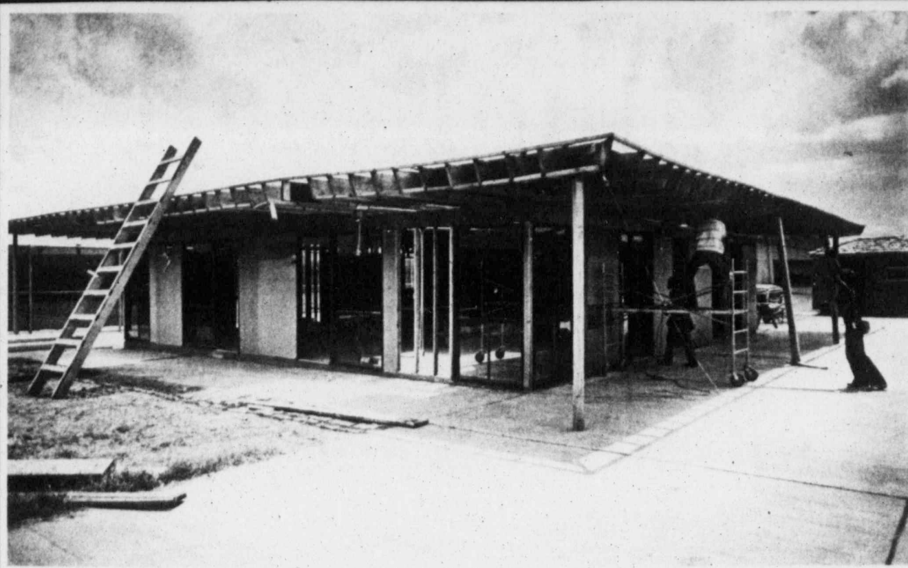
Construction workers Tuesday slide a metal brace on to the roof of the Midland College Tennis Center, as work on the facility resumed. The college hired a second contractor for the project after the first walked off the job last month. Work on the roof and on the inside partitions will have to
