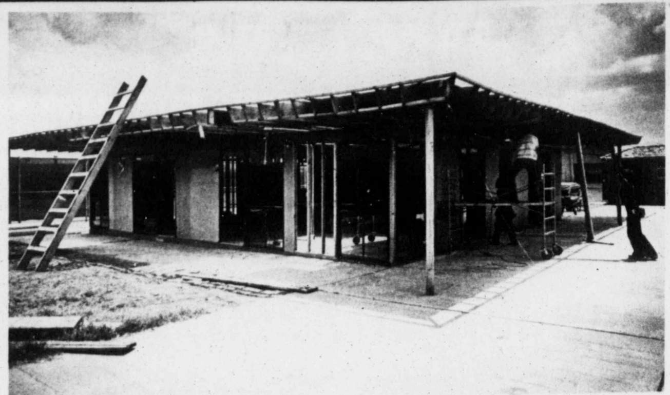
Construction workers Tuesday slide a metal brace on to the roof of the Midland College Tennis Center, as work on the facility resumed. The college hired a second contractor for the project after the first walked off the job last month. Work on the roof and on the inside
