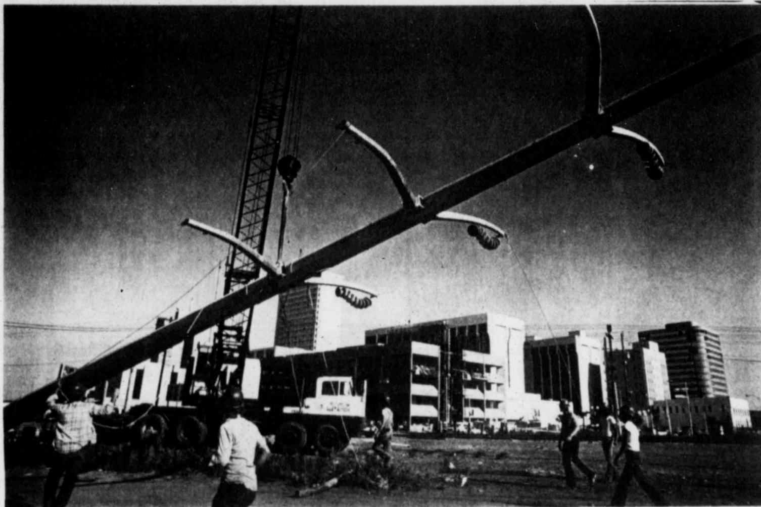
One of 22 structural steel poles that will carry power lines from the new Texas Electric Service Co. substation near downtown to Fairgrounds Road along the Texas & Pacific railway route went up recently. The poles are 80- to
