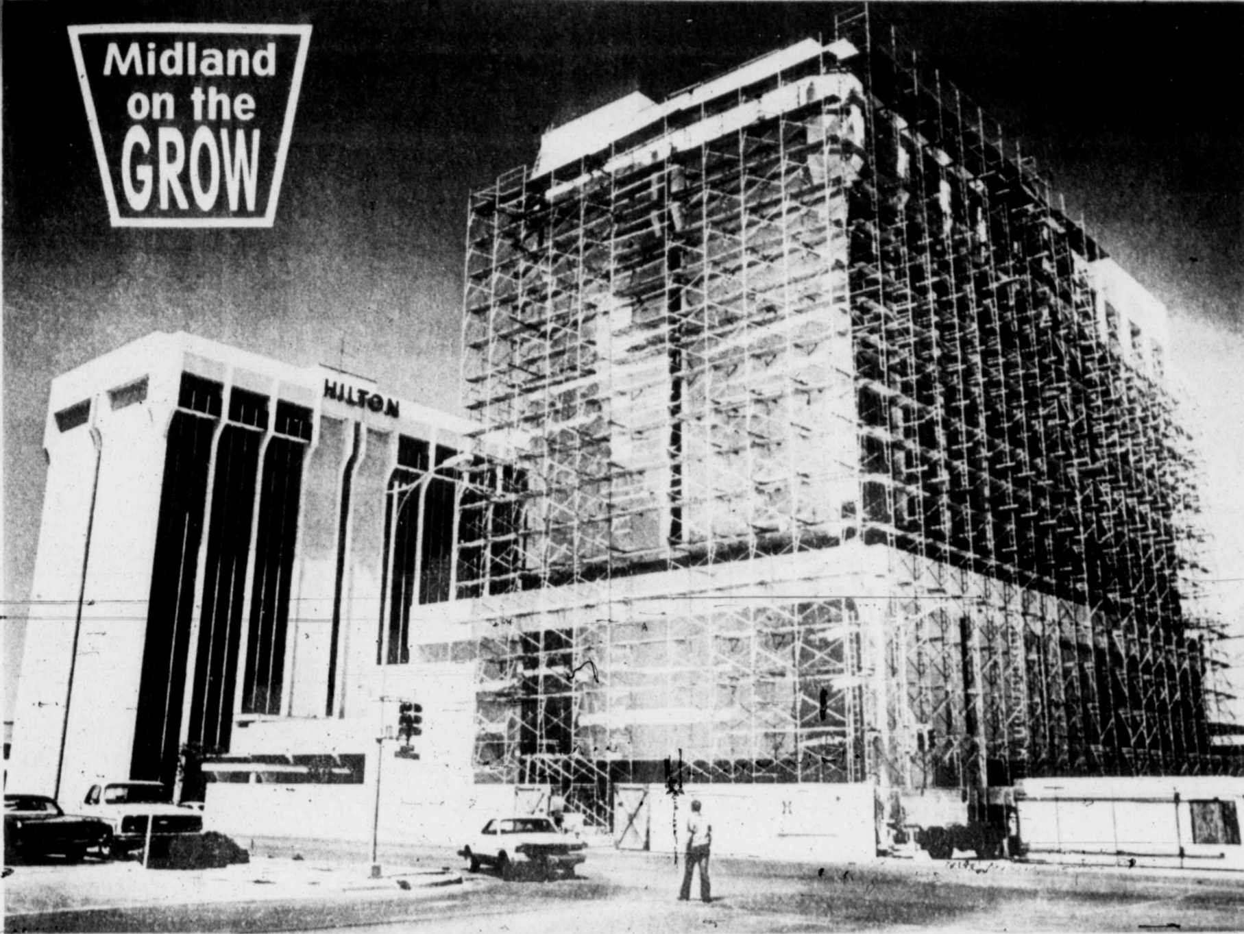
Underneath a beehive-like scaffolding, a "twin" to the Midland Hilton Hotel tower is slowly emerging. When finished, 119 new guest rooms will be added to the hotel, located in downtown Midland at Wall and Loraine Streets. (Staff Photo by Bruce Partain)
