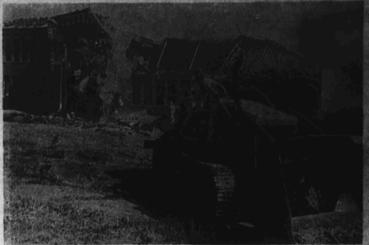
SCHOOLBOY'S DREAM COME TRUE — The walls of a 42-year-old school building at Midland tumble down as Bennie Doggett, Lubbock demolition specialist, fulfills many school-boys' fantasies of how school should really end. Doggett is using a steel cable and tractor to dismantle the building. (AP Laserphoto)
