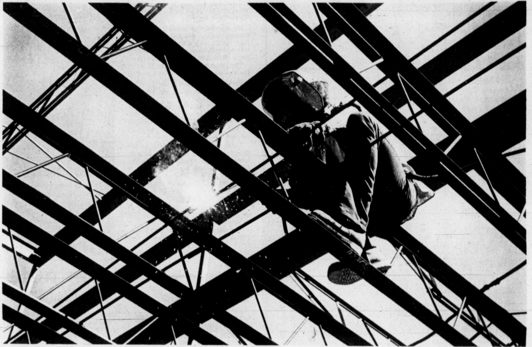
Beginning to take shape after more than four years of planning is the Midland Exhibit Hall on the corner of Main and Wall Streets. Arthur Spurgeon, 24, of Dallas welds cross bars which will make up the ground floor. A piece of Midland history will be preserved within the new building in that part of a turn-of-the-century hotel has been used in the basement structure. (Staff Photo by Mike Kardos)
