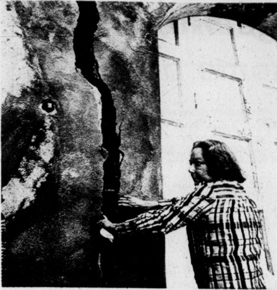
Mrs. Betty Harden looks at the crack between her home and garage in the exclusive Portuguese Bend area where the slow slippage of the ground is damaging many homes in and around the neighborhood in Rancho Palos Verdes, Calif. (AP Laserphoto)
