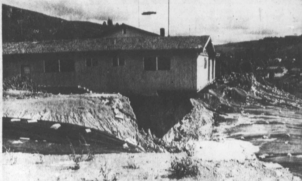
The backyard is slowly slipping away from under this home in northeast San Diego due to the recent heavy rains in the Southern California area. The home has
