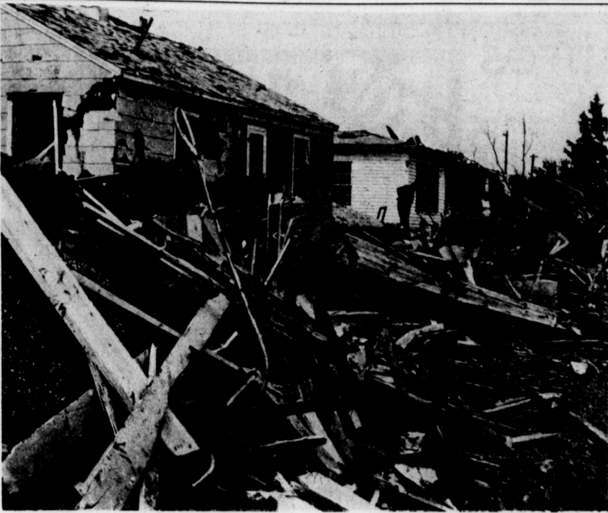
Damage to these two homes in Monahans resulted from an April 1977 tornado, one of the worst to hit this region in recent
