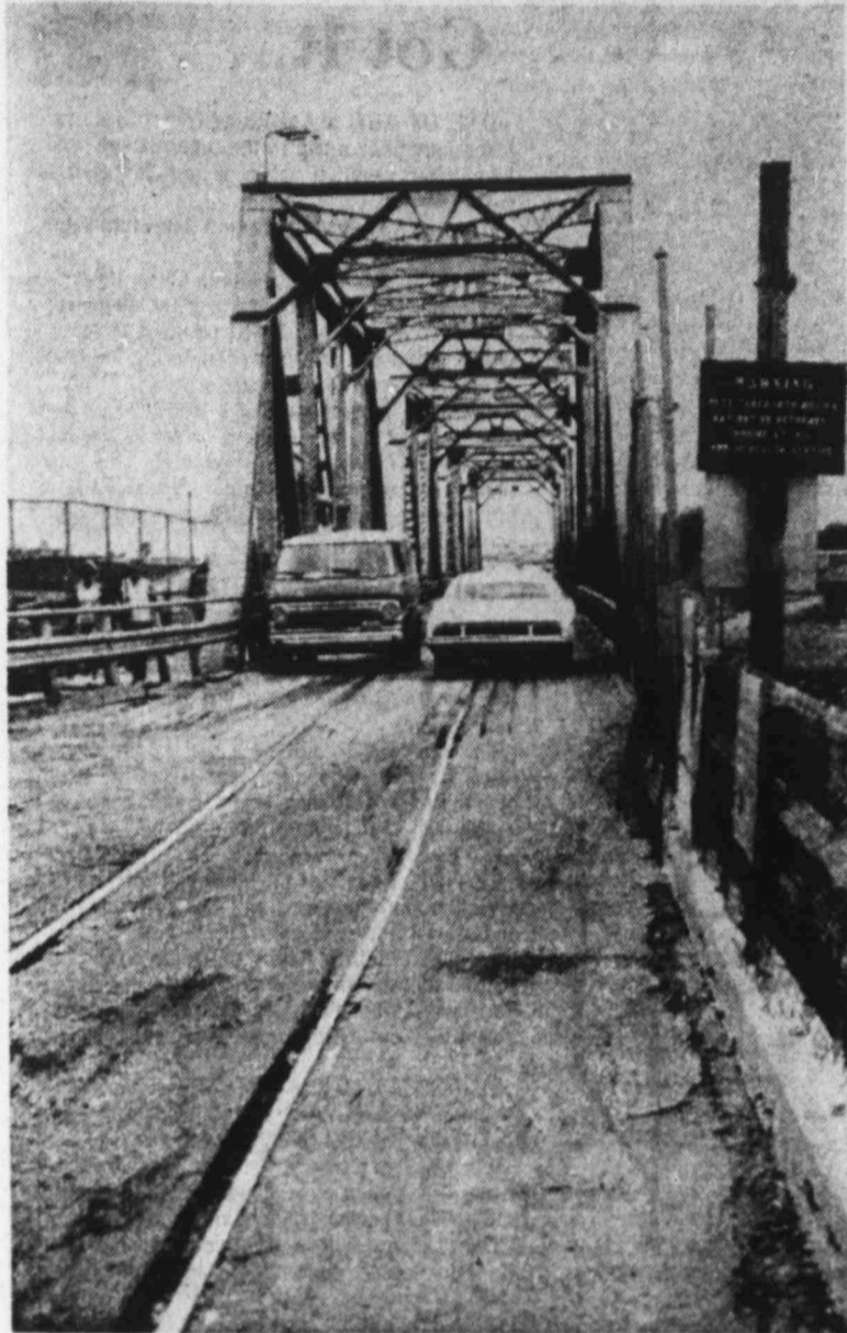
OLD BRIDGE — Traffic on this old railroad bridge connecting Brownsville and Matamoros, Mexico, is halted when freight trains cross the international span. The crossing is one of two often overworked bridges in Brownsville. Officials in the Rio Grande Valley are working toward construction of eight new bridges. (AP Laserphoto)
