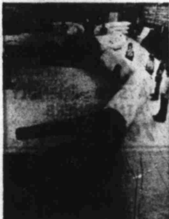
The paper-thin rubberized fabric is black. It gets a coat of white paint. Then it will be painted green.
