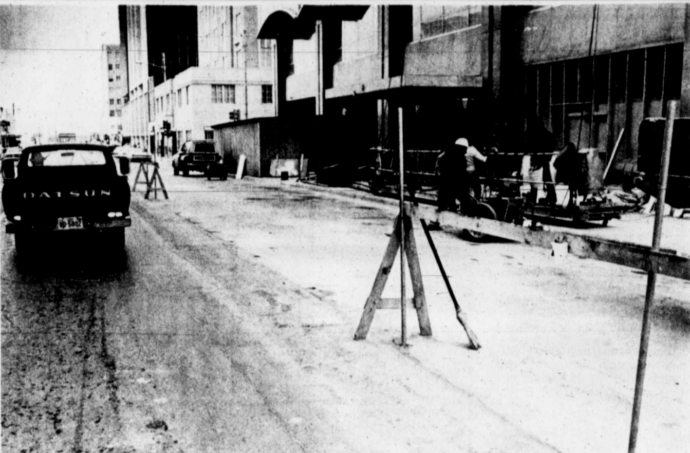
Not for some time have cars and trucks been able to use the right lane of eastbound Wall Street in the downtown area. Tuesday, construction workers removed the barricade in front of The First National Bank of Midland's tower, which is nearing completion. (Staff Photo)
