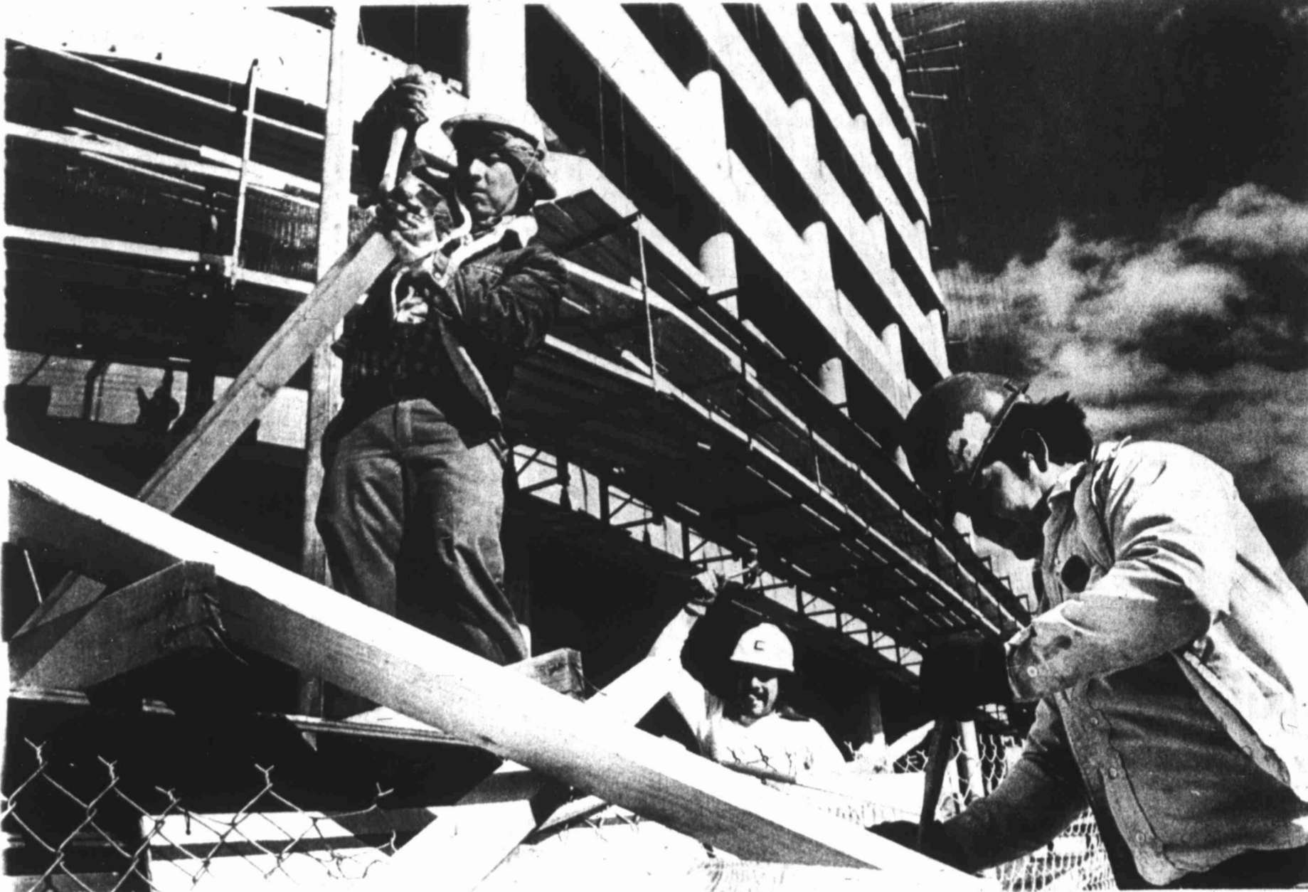
Quannah Construction workers, from left, Salvador Sanchez, Joe Sanchez and Reynaldo Solas disassemble a collapsed section of a passenger walkway just south of the Gibraltar Savings Center on Texas Avenue Wednesday afternoon.
