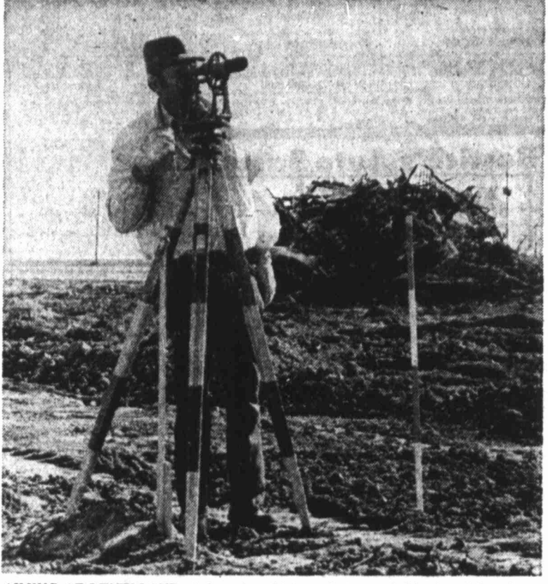
AIMING AT LEVELLAND - A four-lane highway between Lubbock and Levelland comes one step nearer to reality with each sighting down a transit by a Texas Highway Department employee and with removal of piles of debris along the right-of-way for the north lane of SH 114. Trees and structures along most of the route are cleared. (Staff Photo)
