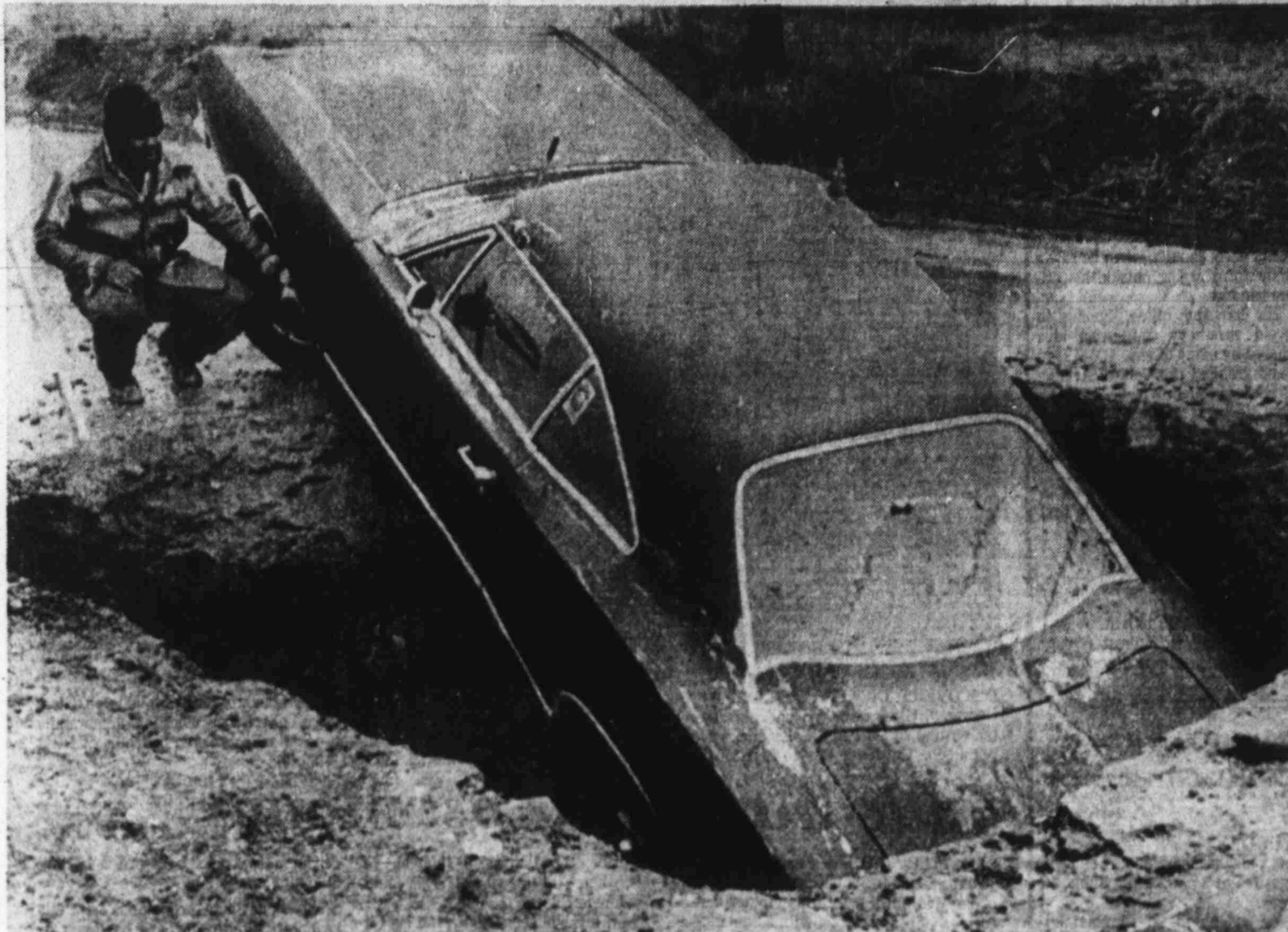
UNDERGROUND PARKING? — Tulsa motorist David Lewis surveys an unusual parking problem after his automobile went out of control and slid backward into a water department excavation. The ditch, over a giant water main, made an icy trap for the vehicle. Freezing rain glazed highways and caused headaches for drivers throughout the northern region of Oklahoma, but few would have willingly traded places with Lewis. (AP Laserphoto)
