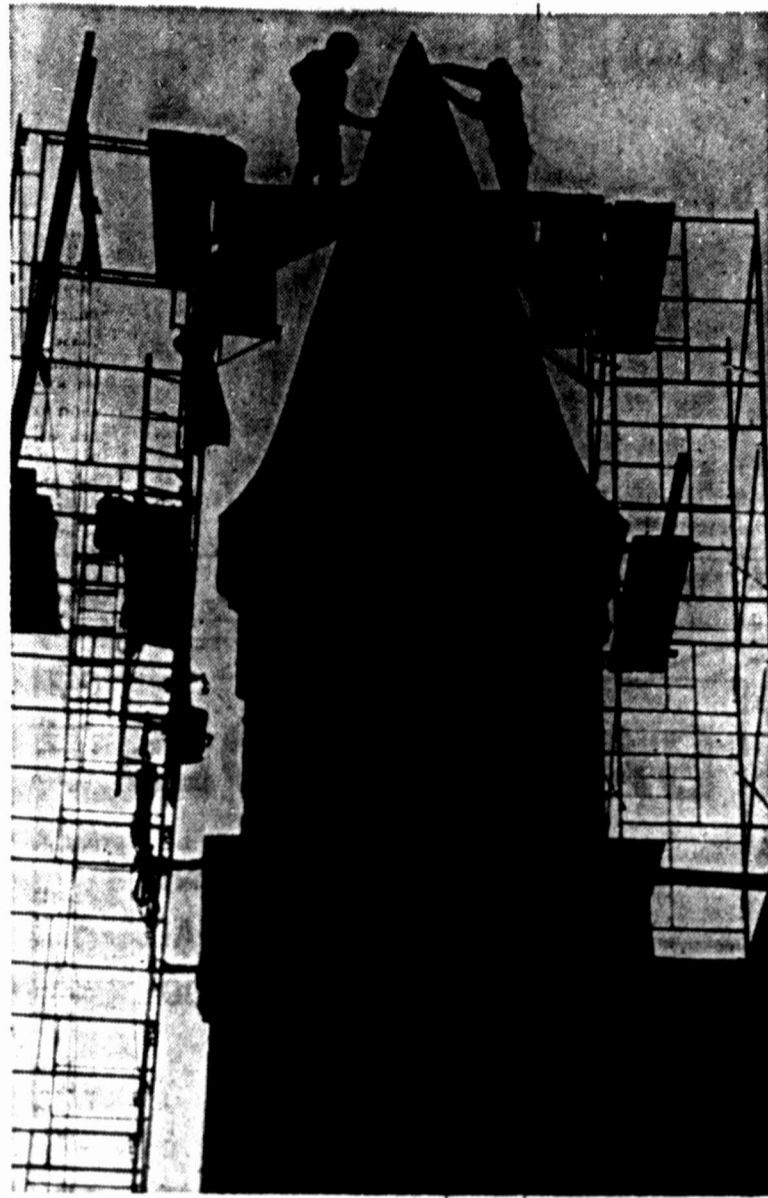
STEEPLE SILHOUETTE — Workers, perched atop scaffolding, repair the steeple of the Black Point Congregational Church in Scarborough, Maine. (AP Laserphoto)
