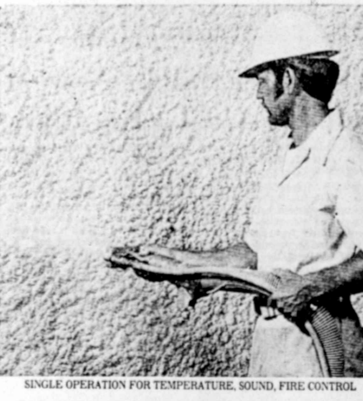
SINGLE OPERATION FOR TEMPERATURE, SOUND, FIRE CONTROL
