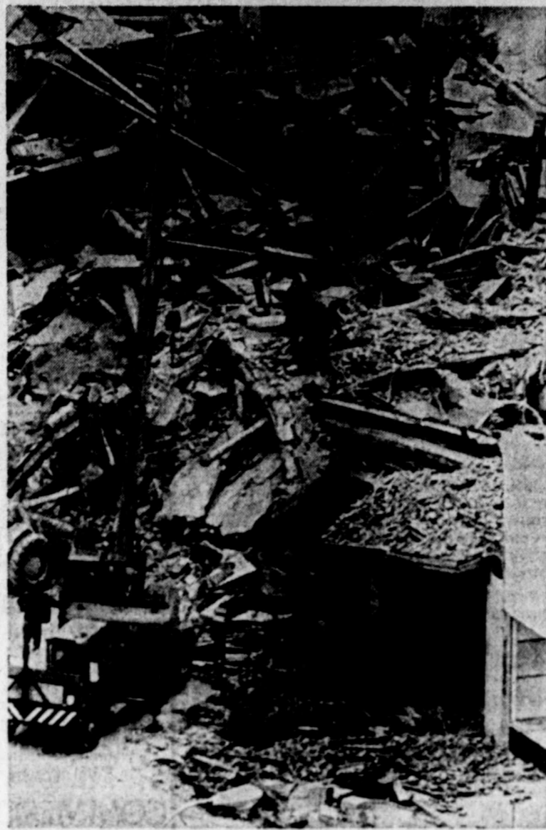
SEARCH FOR BODIES—Rescue workers search for bodies in the debris of the Connor Hotel in downtown Joplin, Mo., which collapsed Saturday as workers prepared the abandoned building for dismantling by means of explosives on Sunday. An unknown number of workers were in the structure when it fell. (AP Laserphoto)
