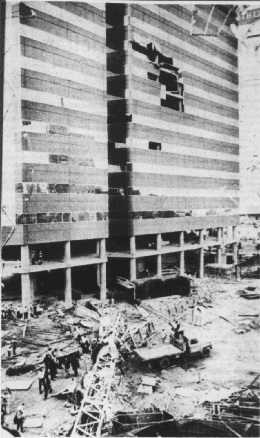
The wreckage of a construction crane litters a downtown Dallas intersection Wednesday after falling 30 stories from the building in the background, killing the crane's operator. The crane smashed into the building on its way down, leaving a large hole in the steel and glass structure. This photo was taken through a window that was shattered by debris from the crane in a building across the street. (AP Laserphoto)
