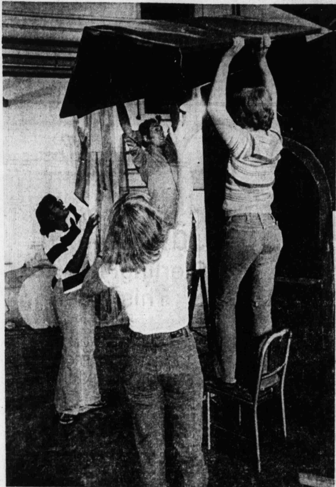
RAISE HIGH THE ROOF — A professional-looking set will enhance the upcoming production of 'La Boheme.' Working on the 'guardhouse' are, clockwise from front, Lucy Tochterman and Veronica Campbell, who are also members of the chorus; Tony Mitchell, stage manager and technical director of the production; and David Morrow, assistant stage director who will perform in the role of 'Parpignol.' Curtain time is 8 p.m. Friday and Saturday. (Staff photo by Holly Kuper)
