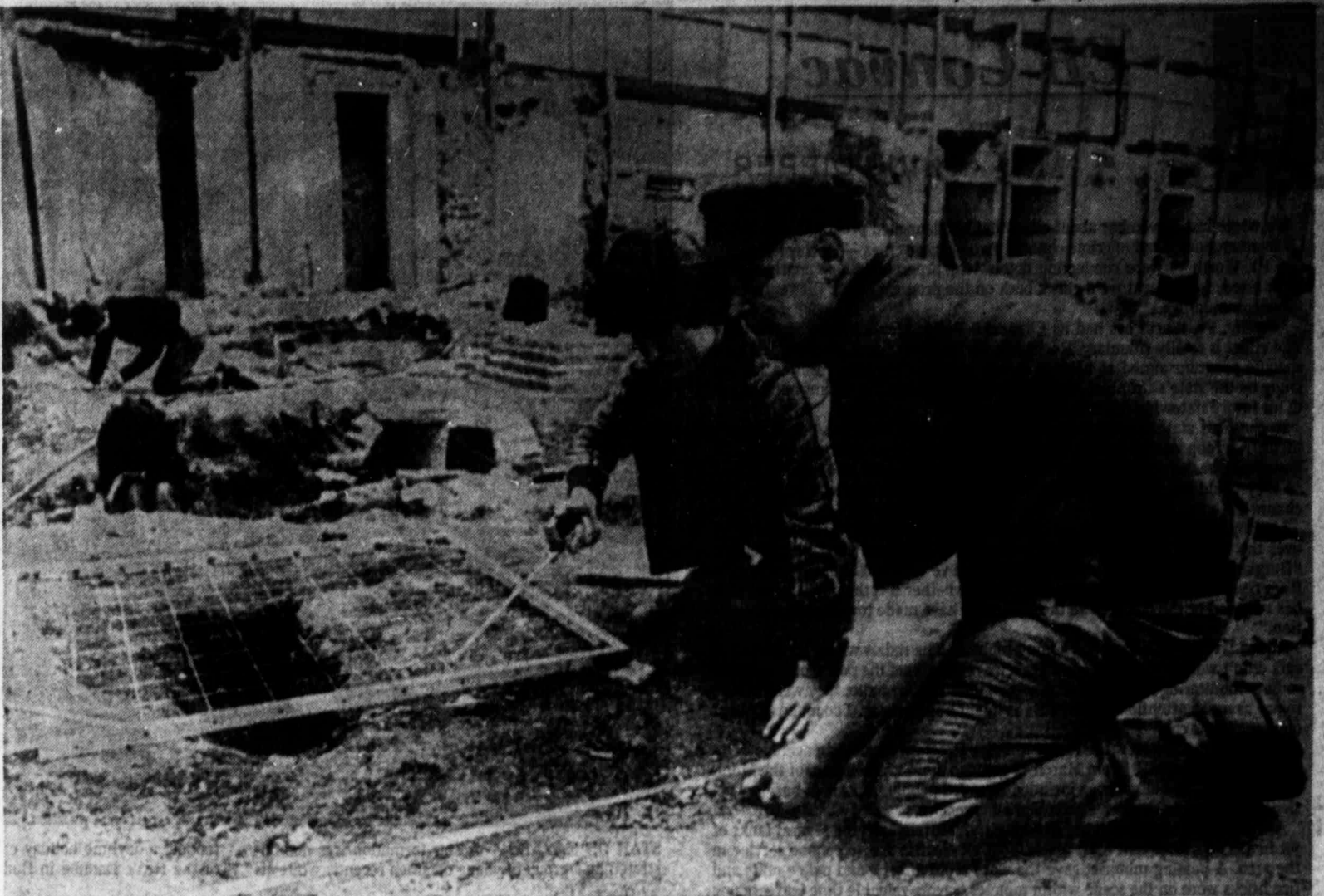
SIFTING THE PAST — Paul Laker of Greenwich, London, and Prof. Glen Ashburn of Western Maryland College, help with excavations on the General Post
