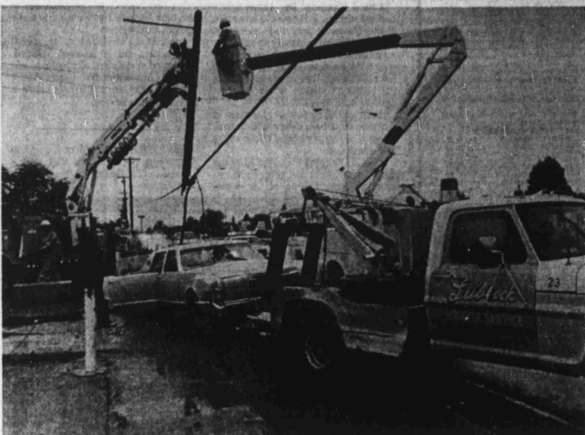
IMPALED ON POLE — Slippery pavement apparently caused this motorist to lose control of his or her car, causing it to slide into a power pole at 26th Street and University Avenue Wednesday night. Southwestern Public Service were called to remove both the broken pole and power lines which stretched across two lanes of traffic. The driver of the car apparently was uninjured in the mishap. (Staff Photo by Gary Davis)
