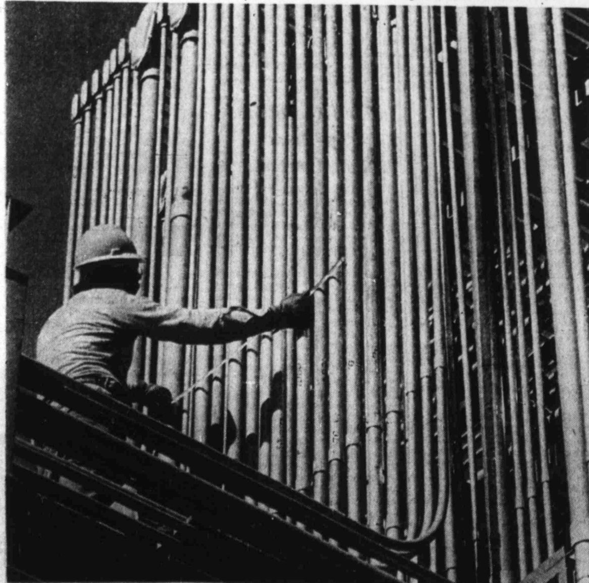
ROOM FOR ONE MORE —Milton Hackfeld, measuring tape in hand, selects a place to put just one more pipe in this crowded field of conduit at the Tenneco Chemicals Inc. plant in Pasadena.
